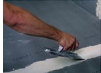
Tape all joints with fiberglass mesh tape or wedi waterproof tape or wedi polyurethane sealant and begin tiling!
